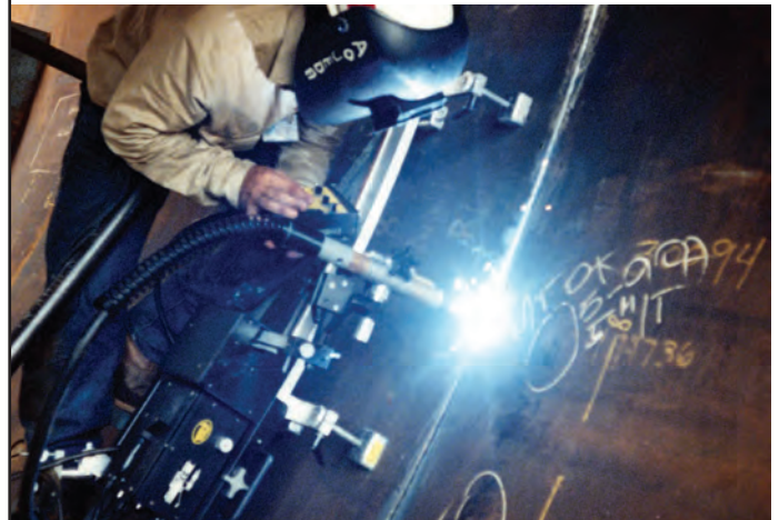
Shown Above - Vertical linear weave welding with ARM-2480 Support Bar w/ Magnets
