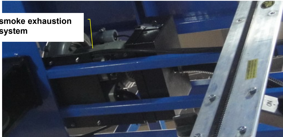
Fig.6. Smoke exhaustion system
